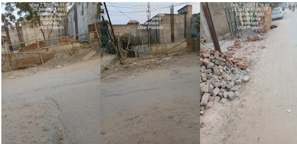
Figure 3.27: Construction material and debris near construction sites
