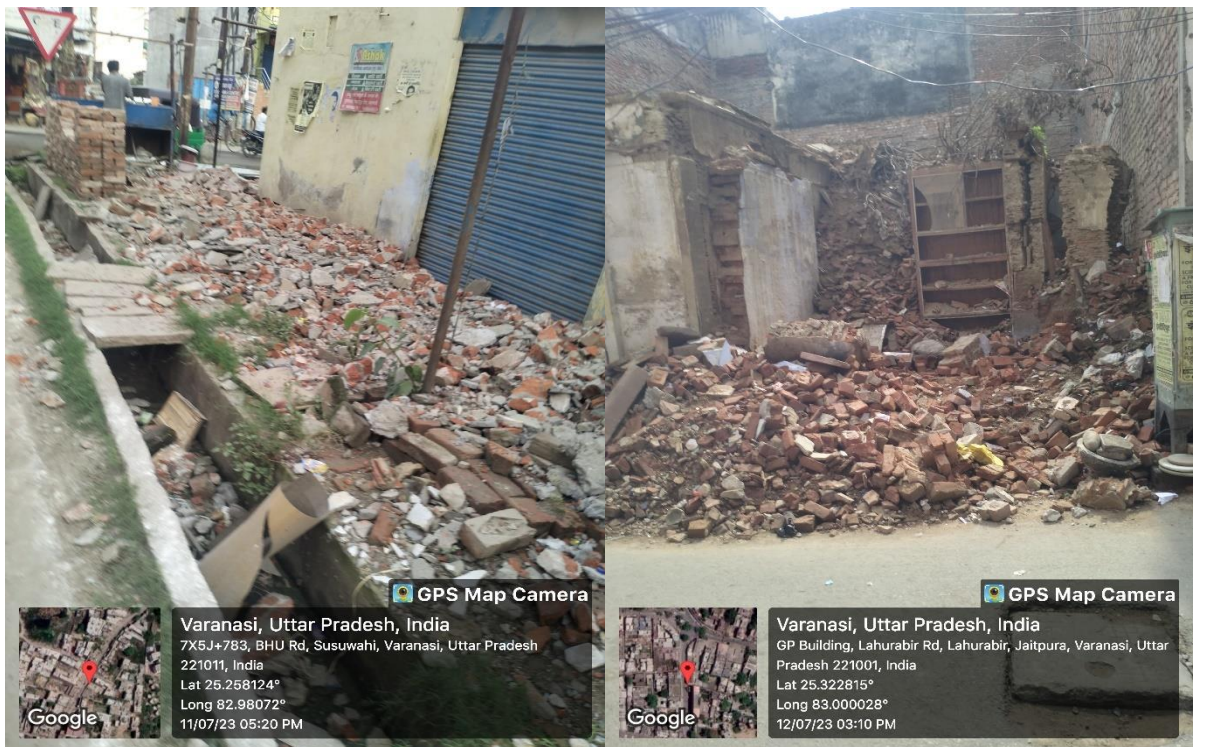
Figure 6.3: Demolition debris near construction sites
