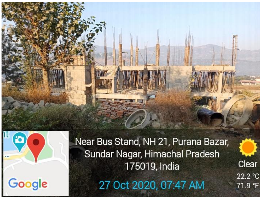
Figure 4.24: Construction material and debris near construction sites
