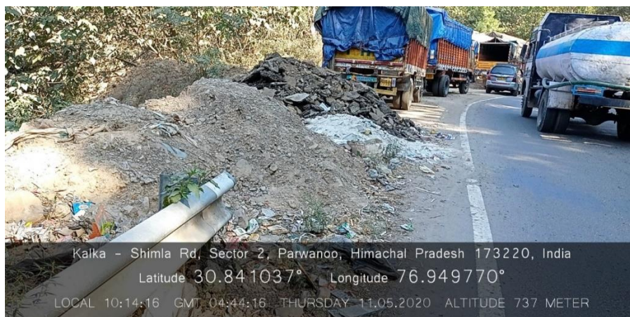
Figure 6.3: Construction material and debris near construction sites
