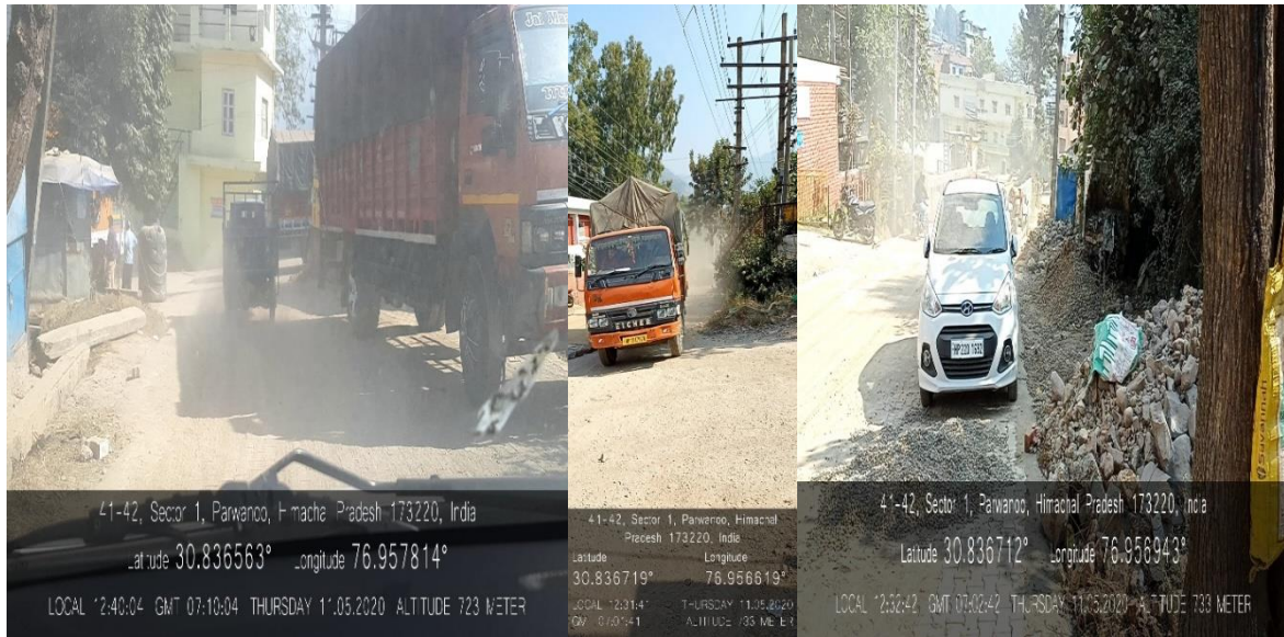
Figure 4.77: Road dust deposition on the paved road
