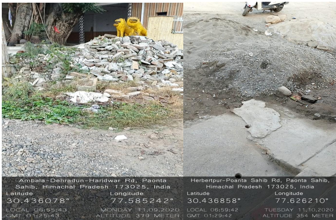
Figure 6.4: Construction material and debris near construction sites
