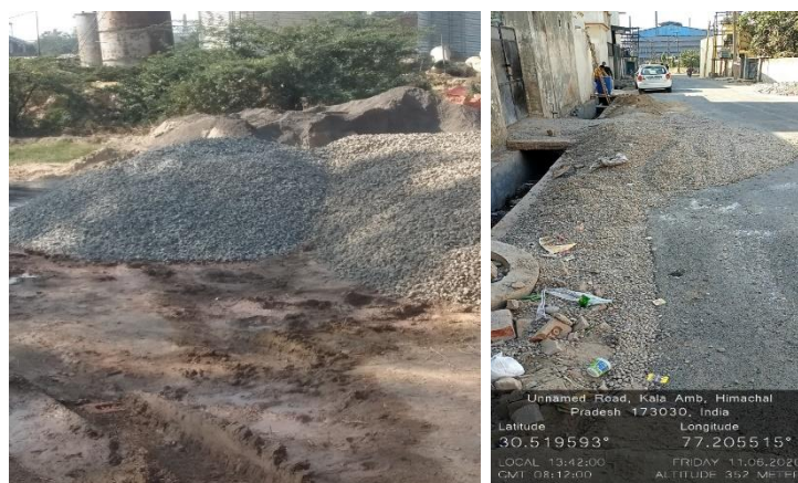
Figure 6.4: Construction material and debris near construction sites
