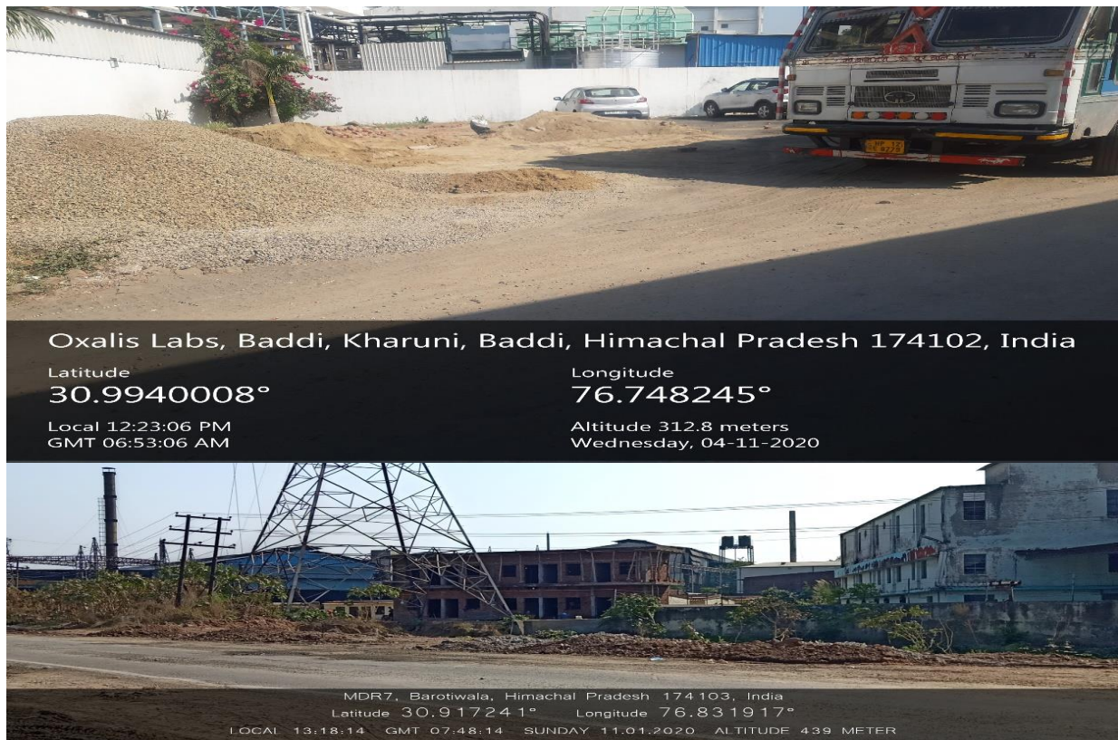
Figure 4.26: Construction material and debris near construction sites
