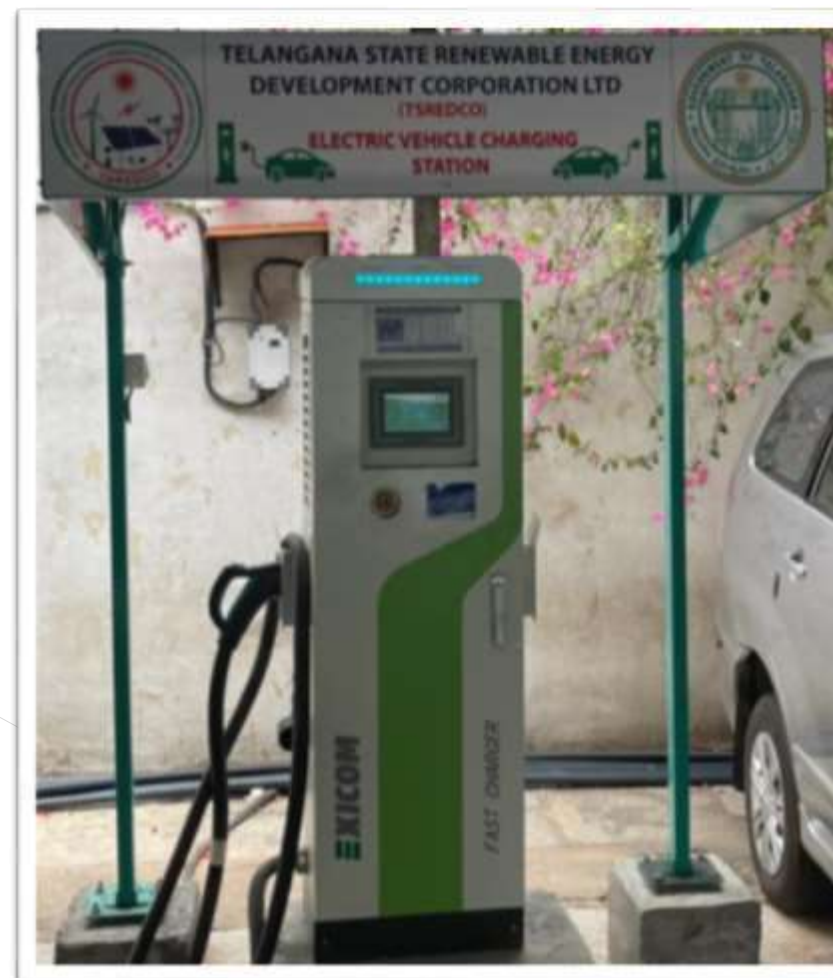
EV charging station @ TSREDCO office
