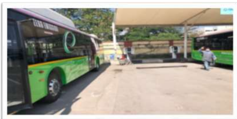
EV charging station @ Jubilee bus station
